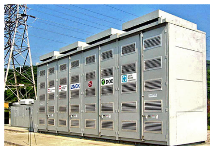
Figure 2 TECHNOLOGY AEP'S NAS INSTALLATION
