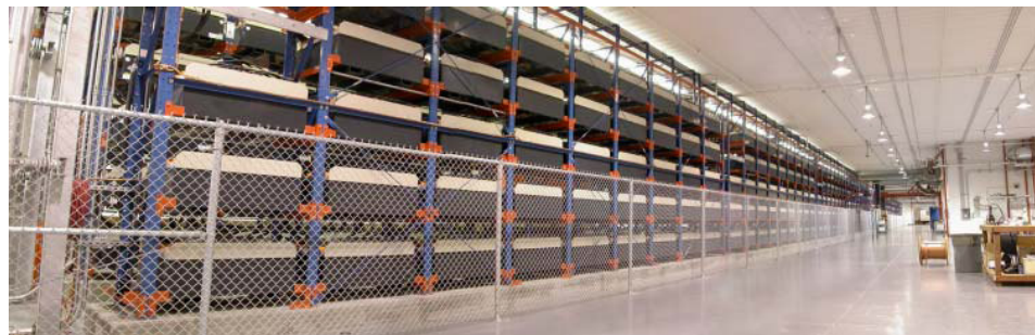
Figure 3 GVEA BATTERY HOUSE
