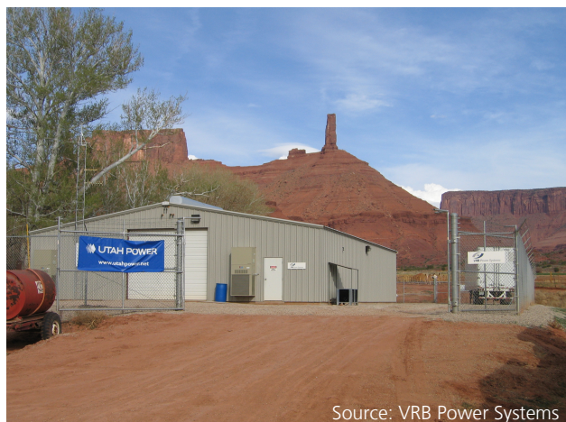
Figure 1 A 250 KW FLOW BATTERY SUPPORTS A UTILITY NETWORK IN UTAH
