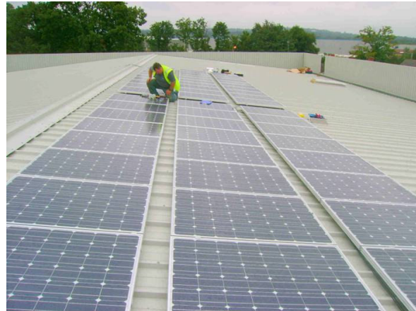
FIGURE 4: A 16 KW PV SYSTEMS INSTALLED ON A WAREHOUSE
